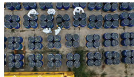
HCH waste and contaminated soil being prepared for transport to incineration sites.
